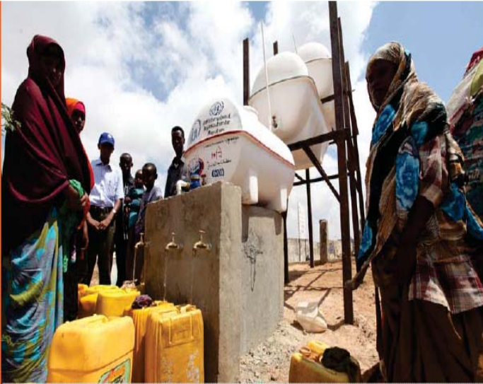
Water treatment facility at one of the camps for internally displaced persons in Mogadishu, Somalia. © IOM 2012
